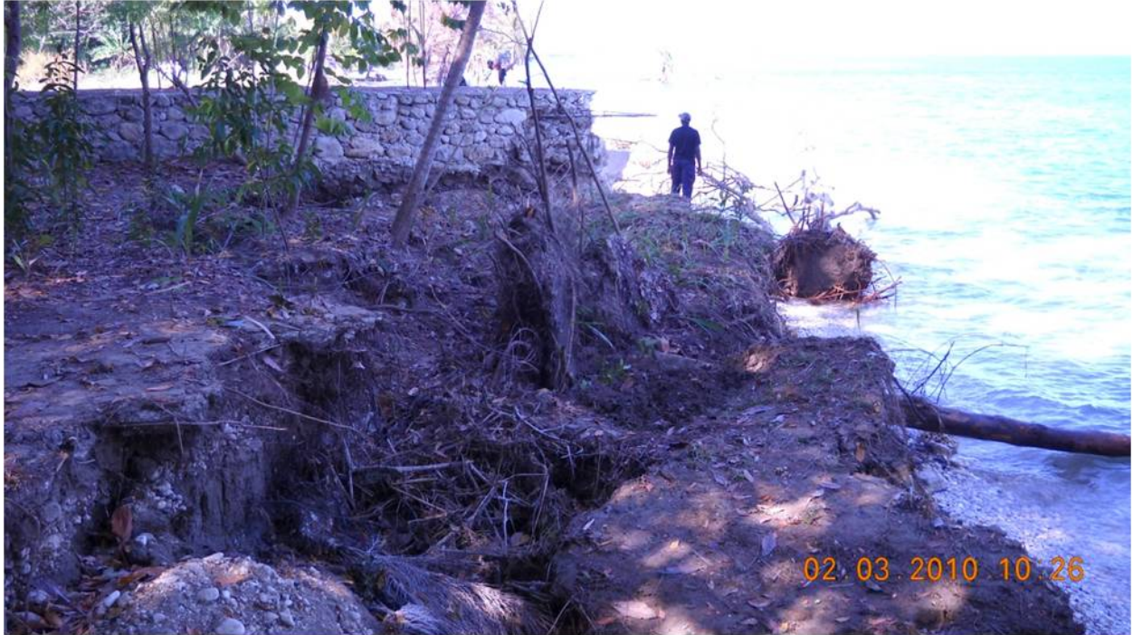
Figure 7.11. Damage to stone wall resulting from coastal failure and lateral spreading. (18°25'33.94"N, 72°43'34.27"W looking westward).
