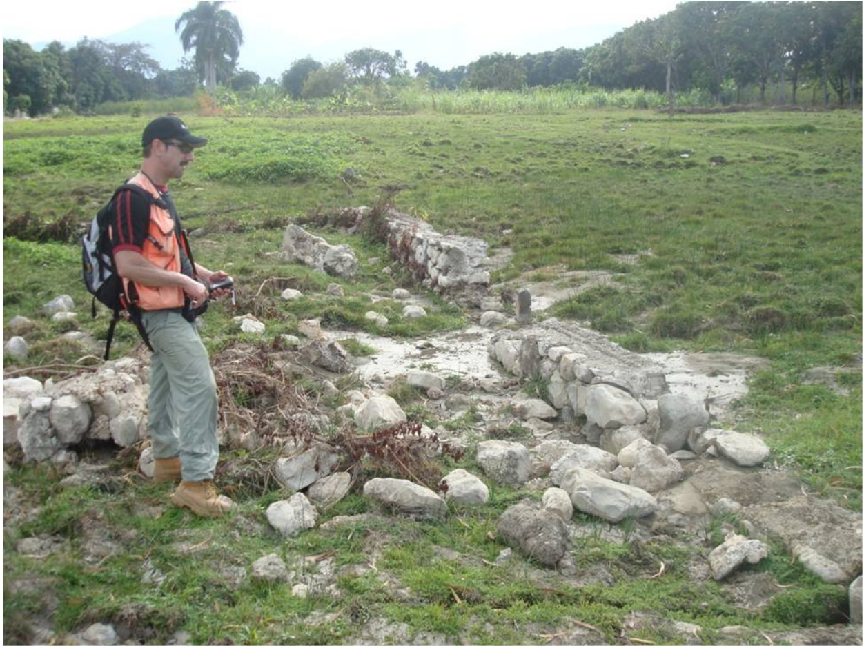
Figure 7.21. Sand blow formation along inland extent of coastal failure near village of Grand Goâve. ( 18^{\circ}25'53.73''\text{N} , 72^{\circ}45'37.65''\text{W} )
