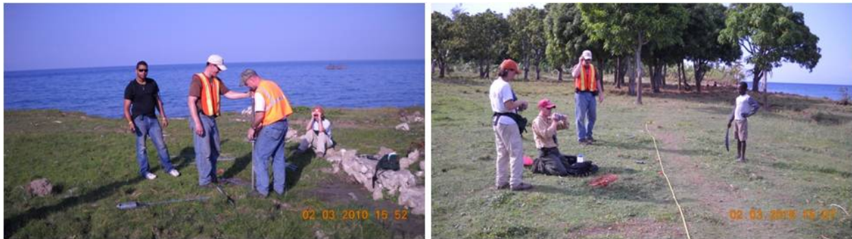
Figure 7.22. DCPT and SASW testing at coastal failure site near village of Grand Goâve. ( 18^{\circ}25'53.64''\text{N} , 72^{\circ}45'37.76''\text{W} for left image, 18^{\circ}25'54.16''\text{N} , 72^{\circ}45'37.85''\text{W} for right image)
