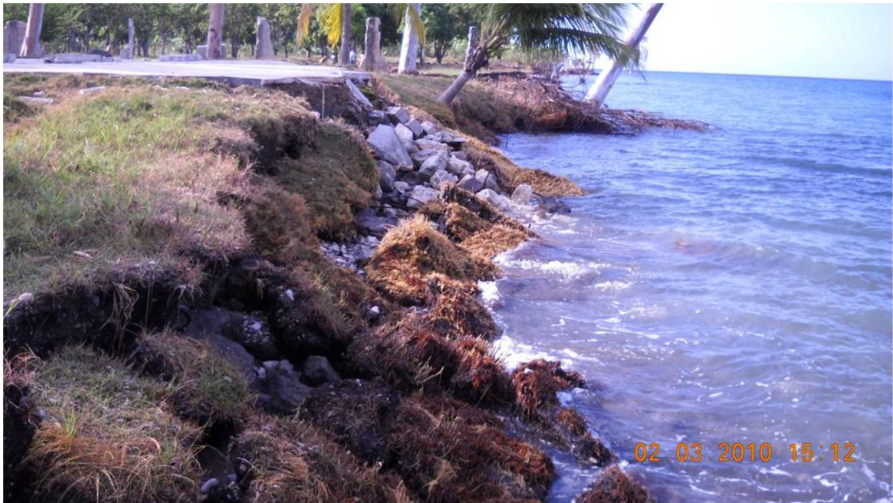
Figure 7.18. Scarp formed along southern portion of coastal failure near village of Grand Goâve. ( 18^{\circ}25'52.91''\text{N} , 72^{\circ}45'35.92''\text{W} looking northwest)
