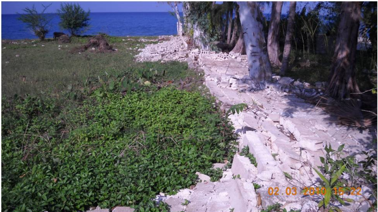
Figure 7.20. Damage to unreinforced block wall running perpendicular to coast near village of Grand Goâve. ( 18^{\circ}25'51.84''\text{N} , 72^{\circ}45'38.06''\text{W} looking northeast).
