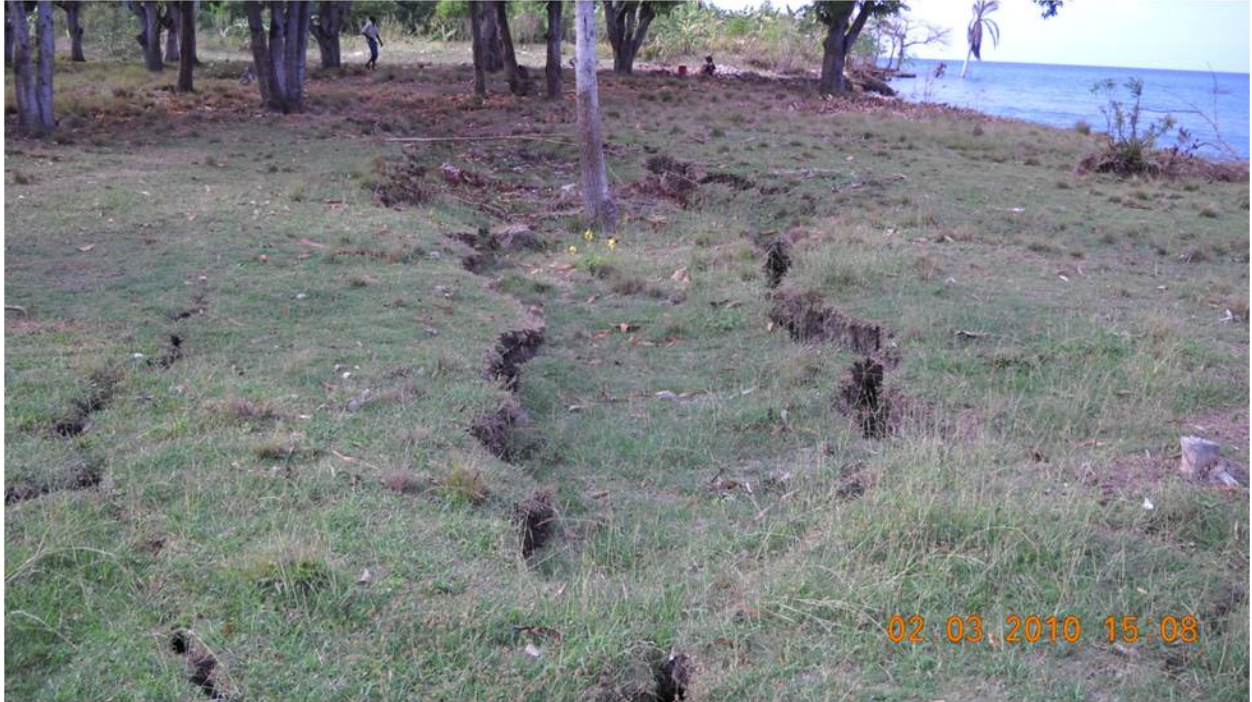
Figure 7.19. Graben formation subparallel to coastline at coastal failure near village of Grand Goâve. ( 18^{\circ}25'54.43''\text{N} , 72^{\circ}45'37.99''\text{W} looking northwest).
