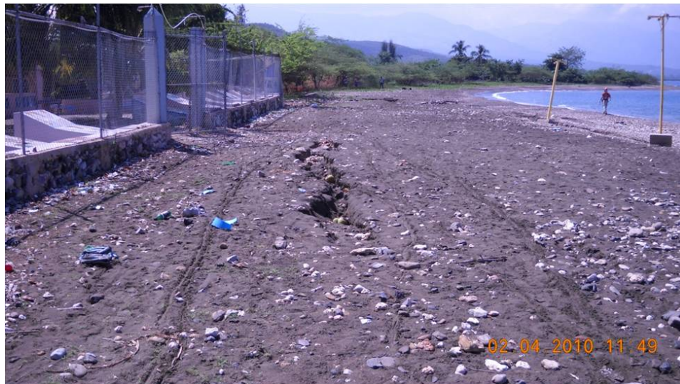
Figure 7.5. Ground cracking along coastline near village of L'Acul. ( 18^{\circ}26'48.83''\text{N} , 72^{\circ}41'11.39''\text{W} looking west).
