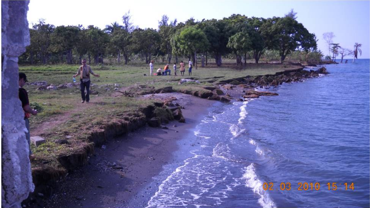
Figure 7.17. Scarp formed along northern portion of coastal failure near village of Grand Goâve. ( 18^{\circ}25'53.82''\text{N} , 72^{\circ}45'37.16''\text{W} looking northwest).
